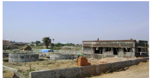
Keelkattalai Main Pumping Station
