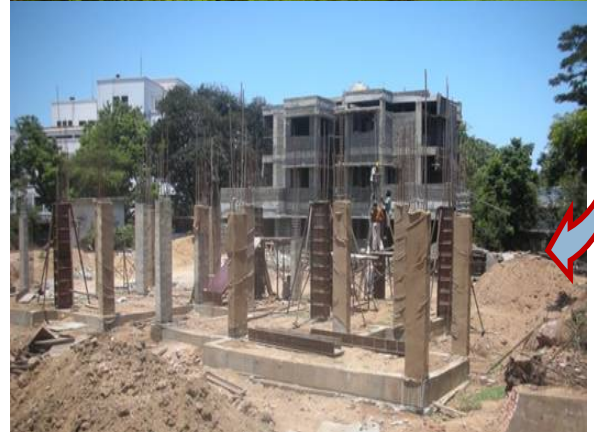
Construction work in the prohibited area
